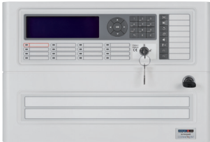
Front view showing key switch fitted
